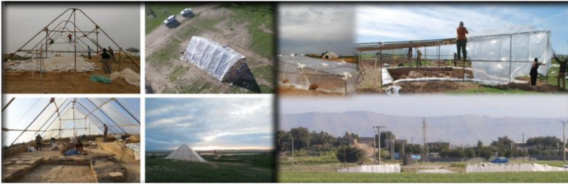
Figure 7. Creating a temporary protective roof for excavation areas in the cemetery and settlement sections of Chega Sofla.
